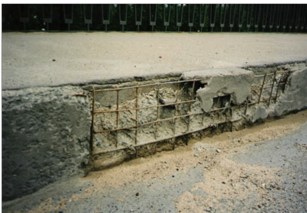
Fig 9. Typical concrete barrier deterioration
