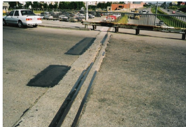
Fig 6. Deterioration of sealed deck expansion joint
