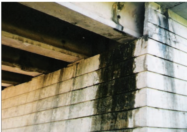
Fig 8. Deterioration of bridge beam ends and abutment due to leakage of expansion joint
