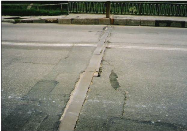
Fig 7. Deterioration of sliding joint
