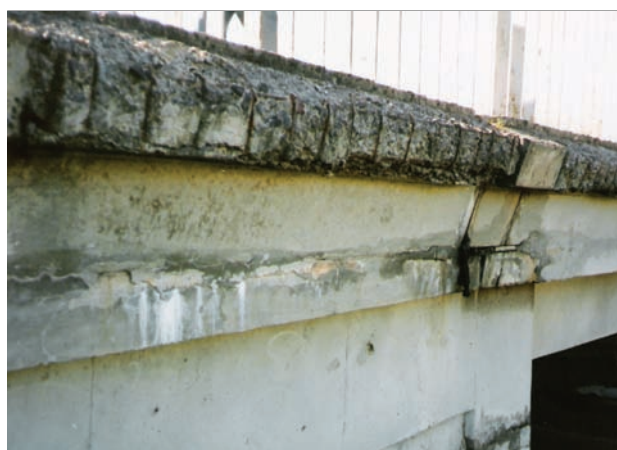
Fig 11. Intensive deterioration along footway deck slab and exterior beam due to seepage of water with de-icing salts from bridge deck
