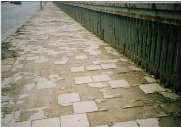
Fig 2. Deterioration of precast concrete overlay in bridge footways
