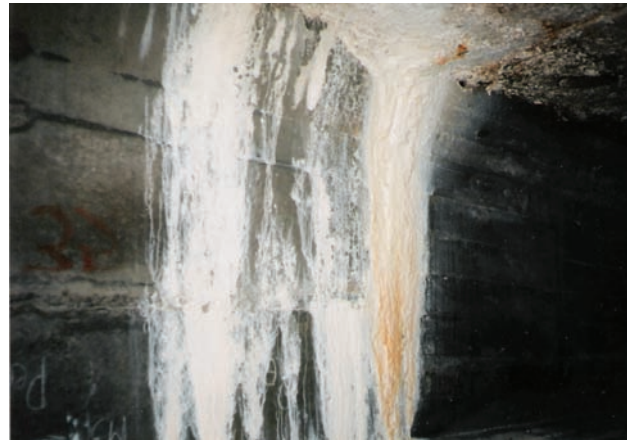
Fig 4. The effect of leaching on the underside of concrete deck of box-girder due to poor waterproofing
