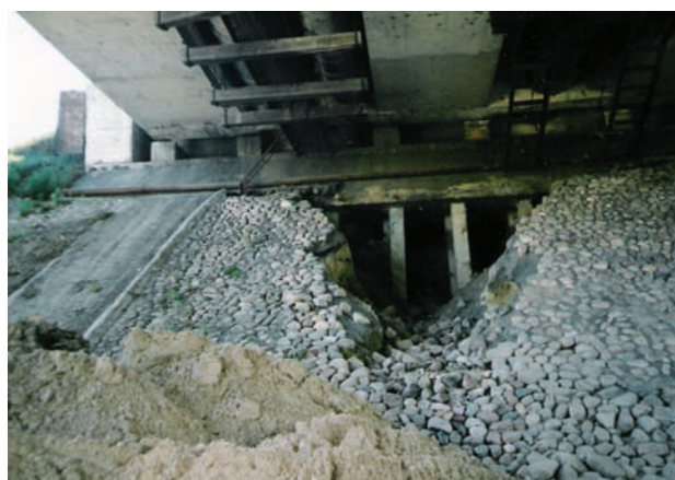
Fig 12. Erosion at the abutment base due to a poor drainage
