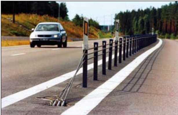
Fig. 2. Wire-barrier on a 13 m wide 3-lane road
