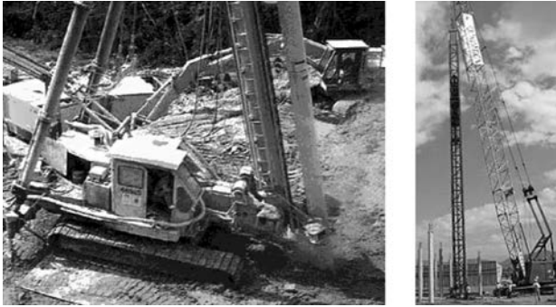
Fig. 4. Inserting circular steel casing into ground by hydraulic hammer mounted on crawler crane
