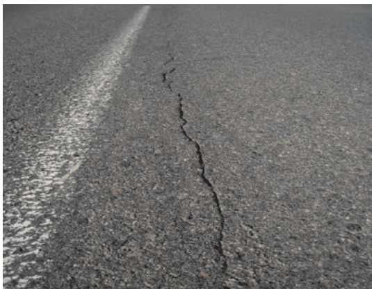
Fig. 10. Longitudinal cracking caused by construction technology violation
