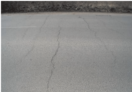
Fig. 9. Transverse cracking in pavement structure with semi rigid surface layer
