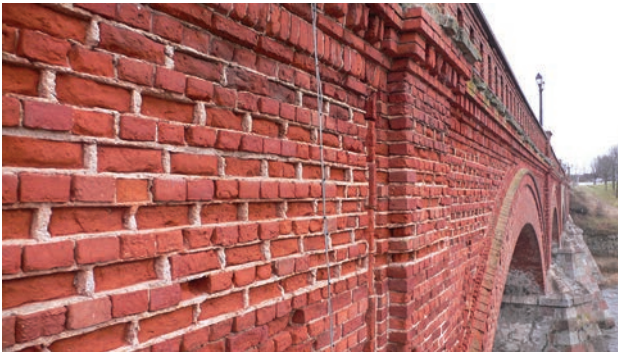
Fig. 5. Corroded and weathered bricks in wall surface from the upstream side
