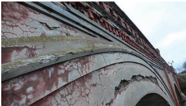
Fig. 6. Cracks and spalling in the reinforced concrete span surface
