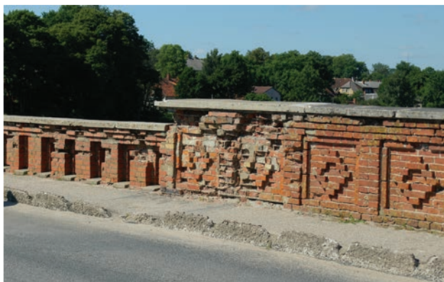
Fig. 8. Serious brick damages in the parapet structure
