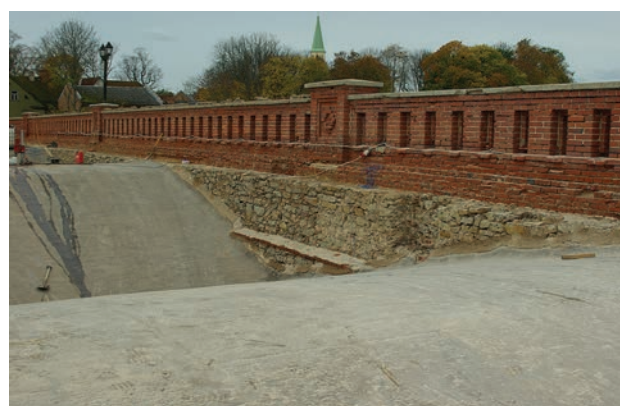
Fig. 10. Opened surfaces of brick arches showed remaining waterproofing and good technical condition
