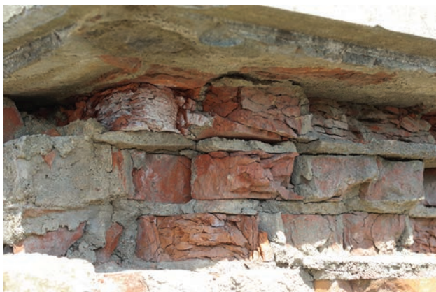
Fig. 9. Disintegrated bricks due to incorrect cladding material selection
