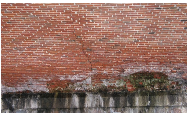
Fig. 7. A crack and falling out bricks around the water drainage pipes on pier 5
