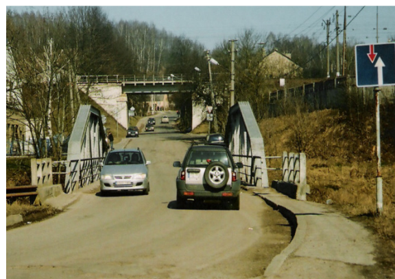
Fig. 2. Urban steel bridge (1930) restricted to one-way traffic in opposite directions: narrow clear roadway (5.8 m) and sidewalks (0.5 m); no shoulders, no sidewalks and lane markings along the bridge
