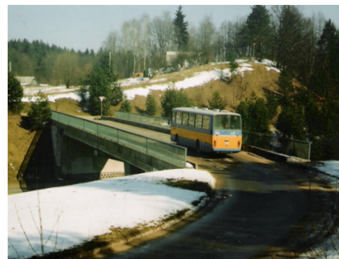
Fig. 9. Example of the bridge on the severe bend in the road and as result with posted traffic speed
