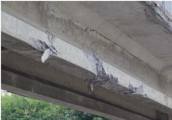
Fig. 5. Collision damage of concrete footbridge with vertical clearance of 4.97 m
