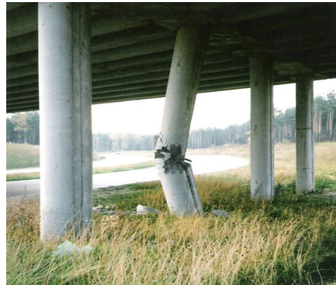
Fig. 7. Collision damage of bridge pier column
