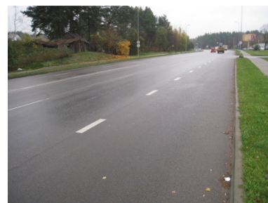
Fig. 2. A view of pavement structure in Geležinio vilko street of Vilnius City in autumn 2012 (6 years after the street pavement structure was laid)
