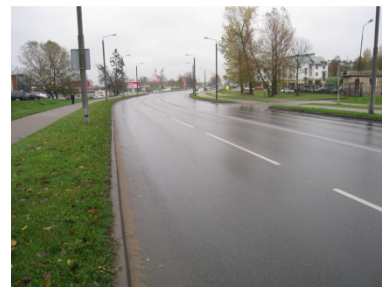
Fig. 1. A view of pavement structure in Ateities street of Vilnius City in autumn 2012 (11 years after the street pavement structure was laid)
