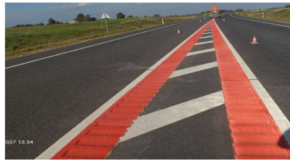
Fig. 3. Rumble strips in the intersection zone
