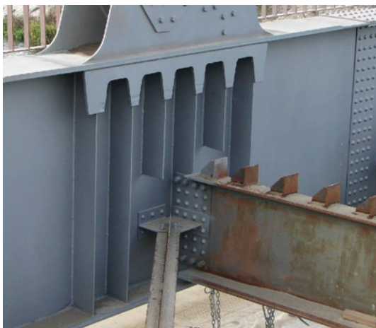
Fig. 3. Example of cross beam to truss girder flange connection; wind bracings gusset plate is visible; picture taken prior to casting of concrete slab
