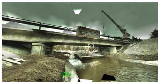
Fig. 4. Full load (1961 kN) placed on the bridge, image view from the scanners position from the Southern side of the bridge
