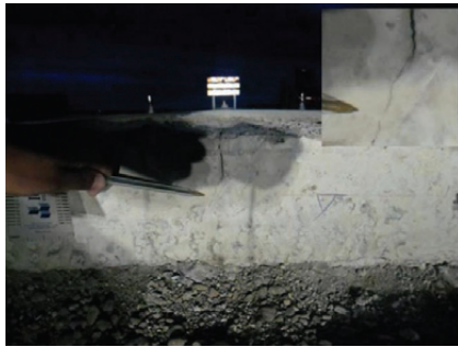
Fig. 2. Crack under longitudinal joint in JPCP (7 m width), Tierra del Fuego Province. 2:00 am – temperature at the surface of the pavement 10 °C
