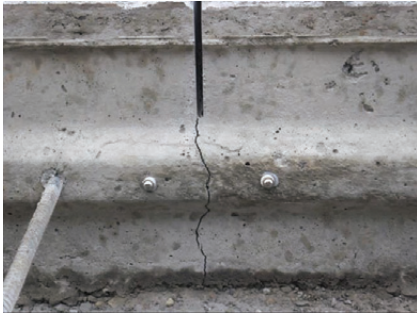
Fig. 1. Crack under transverse joint in JPCP, Province of Concepcion. 8:00 am – temperature at the surface of the pavement 13 °C
