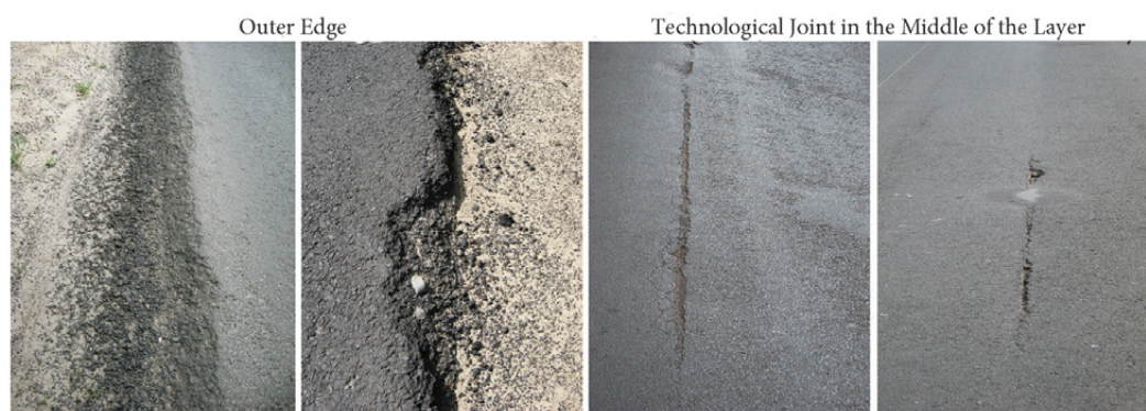
Fig. 1. Damage on the asphalt surface in the area
