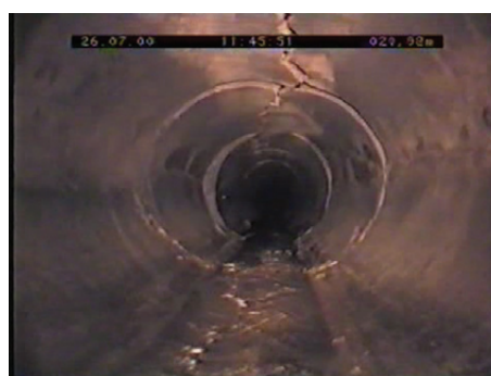
Fig. 4. Vertical deformation of a cracked pipe
