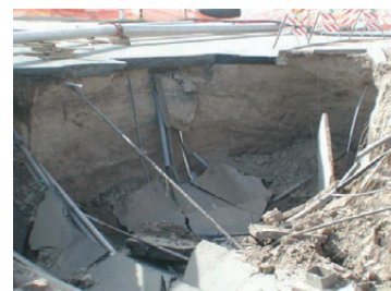
Fig. 2. Road pavement collapse with visible damaged cables and pipes
