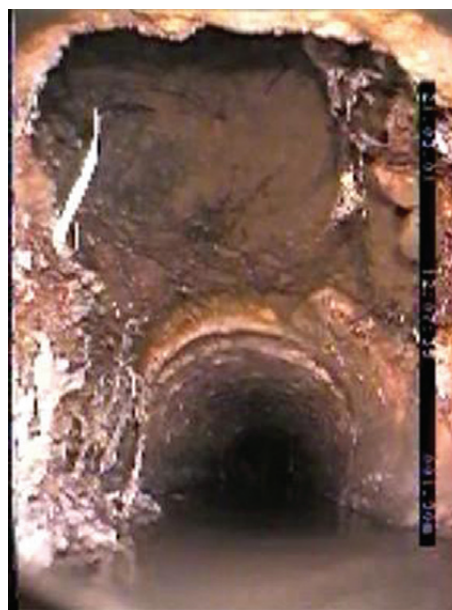
Fig. 5. Sewer collapse, an air void visible above the missing fragment of the sewer wall
