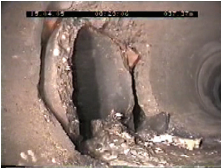
Fig. 7. Defective connection with visible air voids beyond the sewer wall
