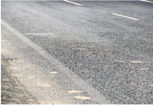
Figure 2. Ravelling on pavement section NH-8GJ at 434.00 km
