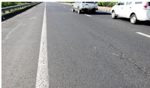
Figure 1. Surface condition evaluation on pavement section NE-1GJ02 at 32.00 km
