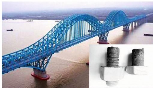
Figure 1. The Dashengguan Railway Bridge and bolt fracture
