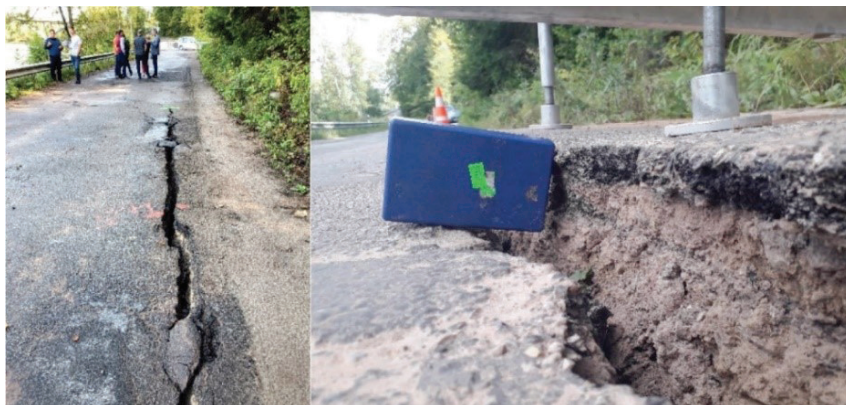
Figure 3. Deformations on existing roads
