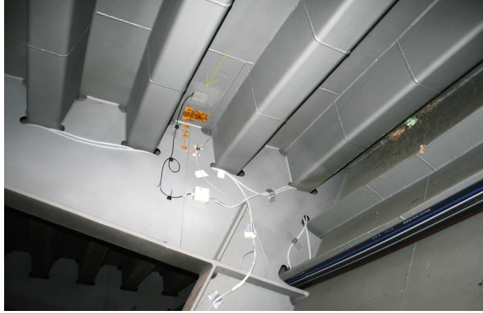
Figure 8. Photo of girder interior (connection of the top slab with external slanted wall), arrow shows point-wise temperature sensor of the top slab T_3
