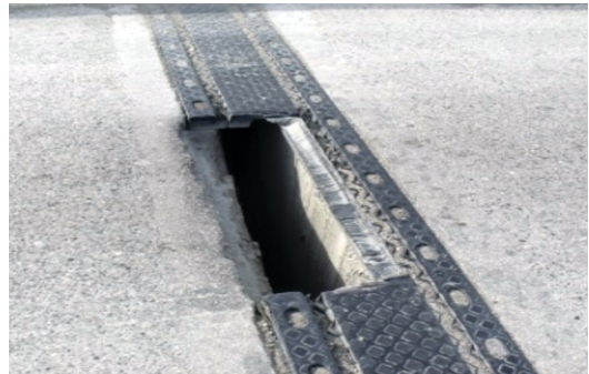
(b) Partly missing expansion joint
