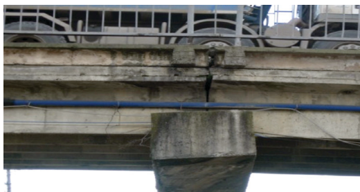
(a) Wrong connection and slope
