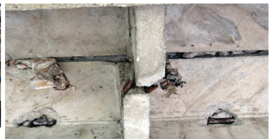
(b) Poor workmanship misalignment
