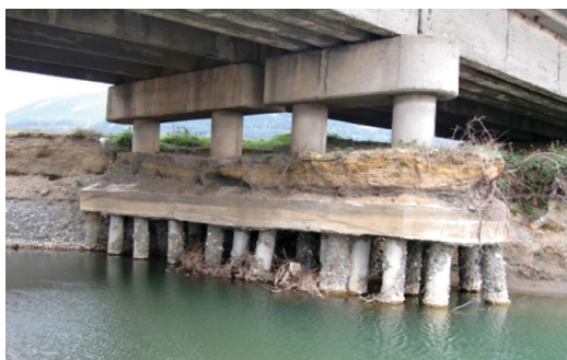
(a) Heavy scour
