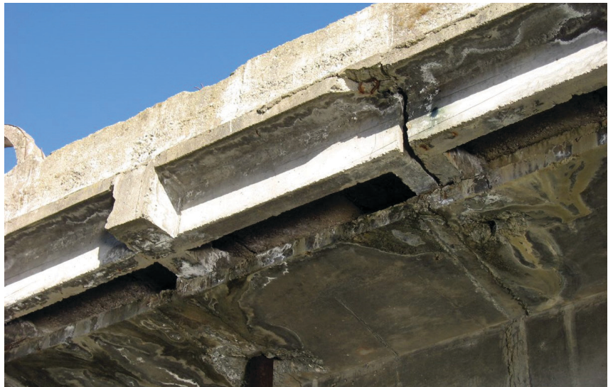
Figure 7. Chemical attack on a reinforced concrete bridge
