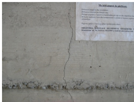
(c) Plastic shear crack at abutments
