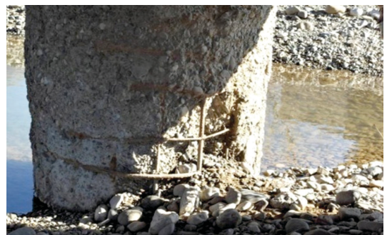
(b) Exposed steel bars
