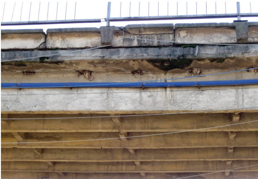
Figure 19. Parapet defect on reinforced concrete beam
