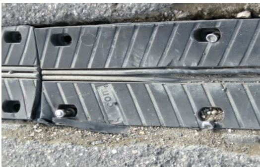
(a) Out of function expansion joint
