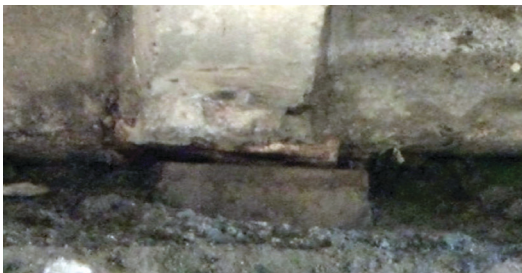
(b) Misalignment of sliding bearing
