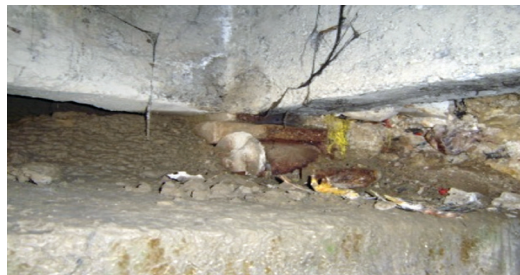
(a) Corroded and clogged bearing
