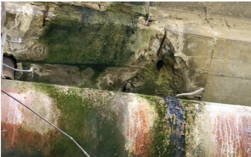
Figure 9. A typical water leakage
