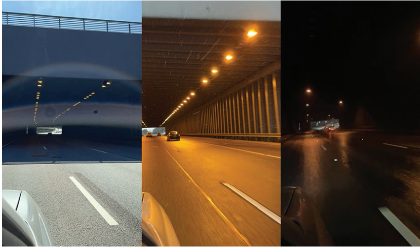
Figure 7. Lighting of Gudeliai tunnel under different conditions (from left to right: sunny, cloudy and night)
