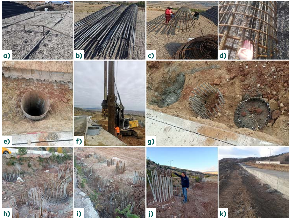
Figure 10. (a) Reinforcement workbench set up in the inspection area; (b, c, d) Preparation of reinforcements with stirrups and steel ties; (e) Circular section drilling for bored pile application; (f) Placement of steel reinforcement in the bored pile hole; (g) Formation of bored piles; (h, i) Application of the bored pile work with two rows; (j, k) Reinforcement and concrete of the cap beam
