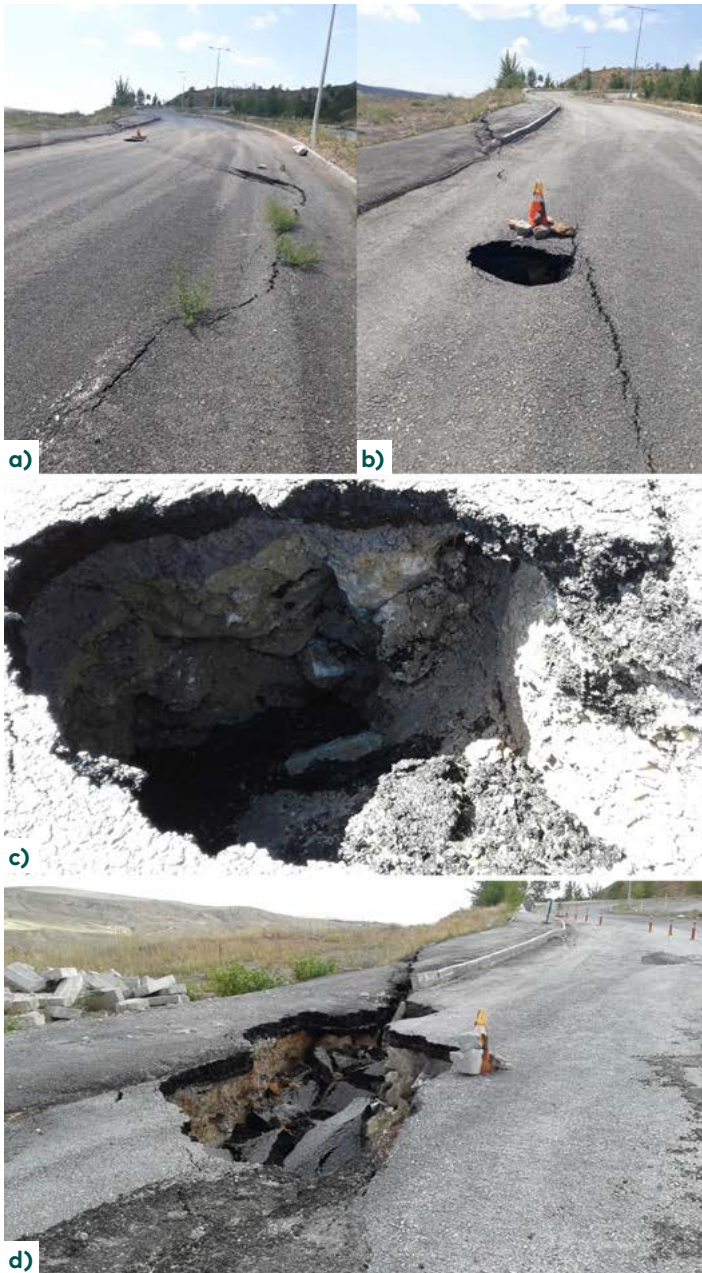
Figure 5. (a, b) Collapse and cracks-fissures on the Ulu yazı campus road surface; (c, d) collapse pits
