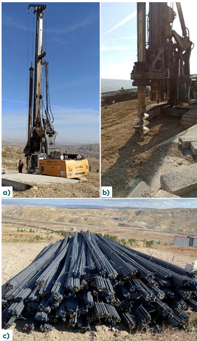
Figure 9. (a, b) Drilling work related to bored pile works in the field, (c) Bringing the bored pile reinforcements to the study area
