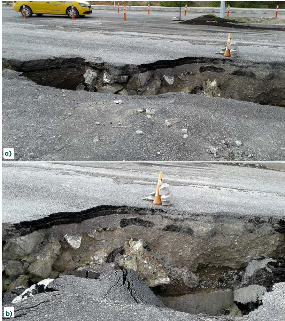
Figure 4. (a, b) Gypsum block filling material of the road infrastructure in the collapse pits and aggregates used in the road superstructure
