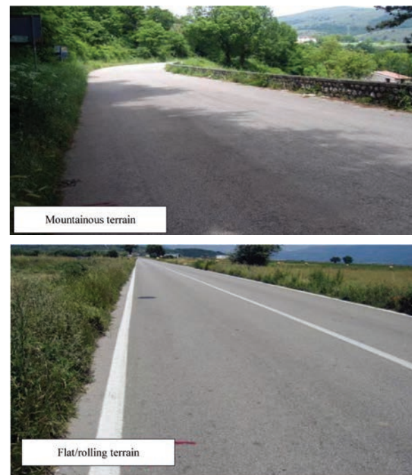
Fig. 1. Photographs of a typical road located on the mountainous and flat/rolling area
