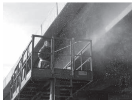
Fig. 1. Repair of road bridge in Brno (Czech Republic) using hand-held water jet lance tool
